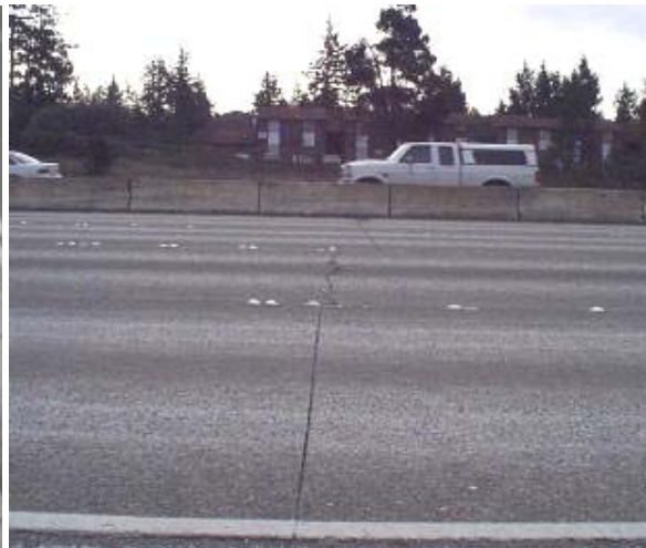
Figure 2.26: Missing Contraction Joint (The middle lane contraction joint was not sawed resulting in a transverse slab crack. The outer lanes have proper contraction joints and therefore, no cracking)
