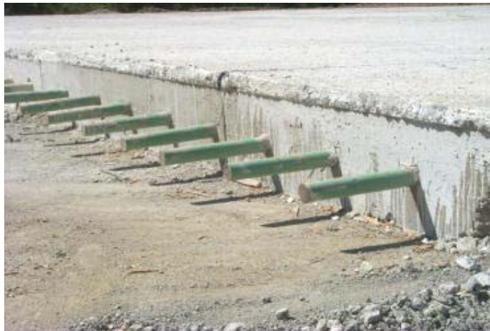
Figure 1.26: Dowel Bars in Place at a Construction Joint- the Green Color is from the Epoxy Coating
